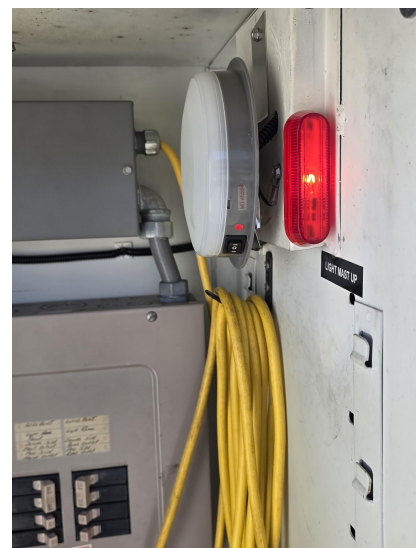
Mast Warning Light #2 is located in Compartment #2 on the right side wall.
